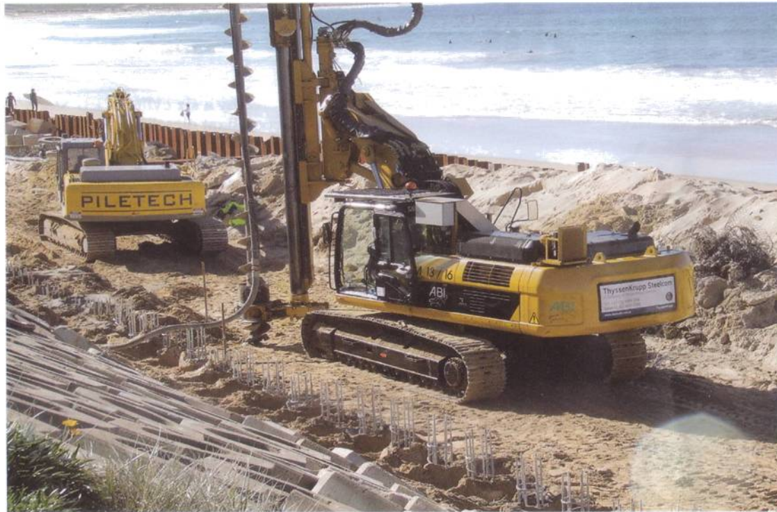
The ABI rig requires half the personnel and takes less space compared to a crane, power pack, hoses and hammer.
